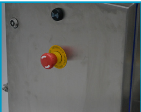
Dual Emergency Stop buttons, accessible from both sides of the line
